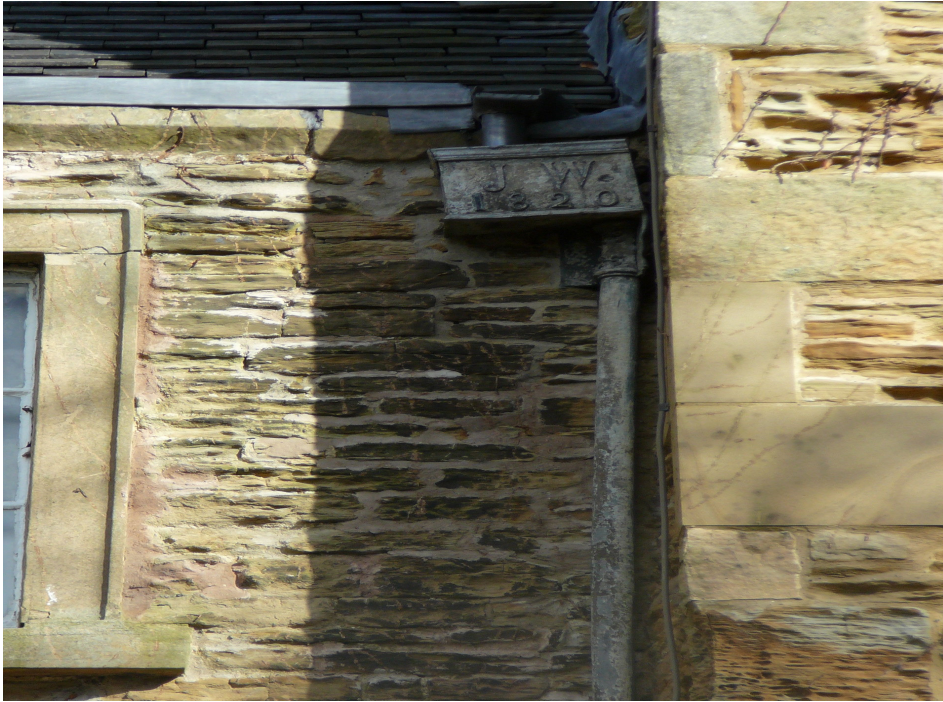
Carnfield Hall – detail of wall showing both Coal Measures sandstone & Magnesian limestone. Note also the hopper inscribed 'J.W. 1820'.
