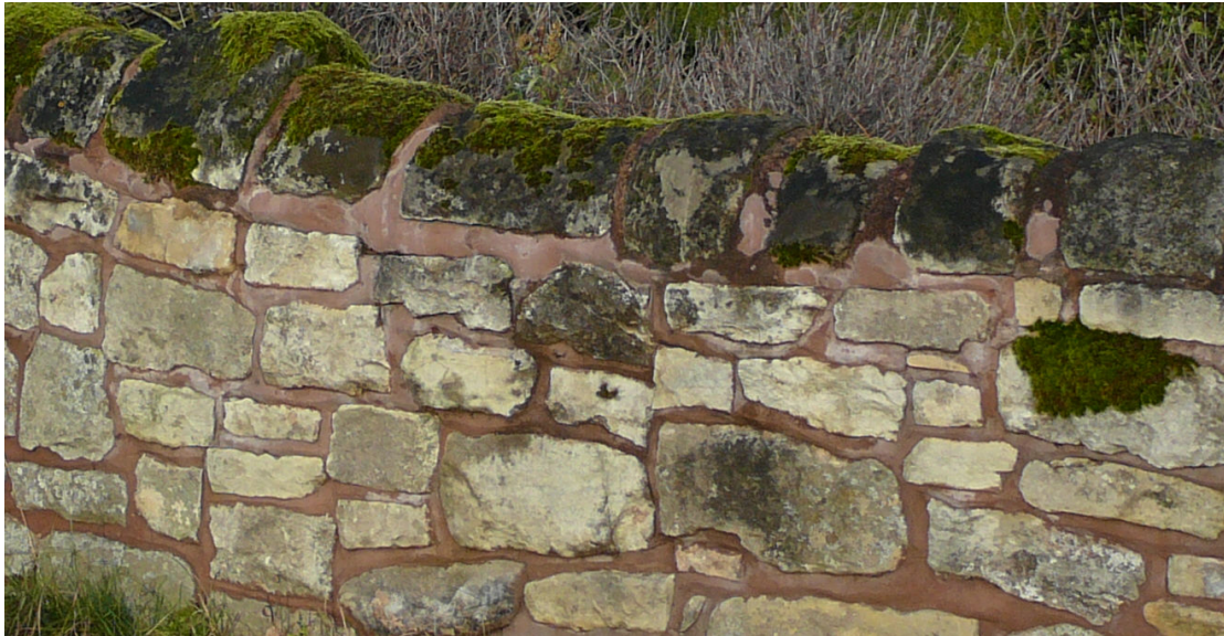
Example of inappropriate pointing using cement-based mortar
