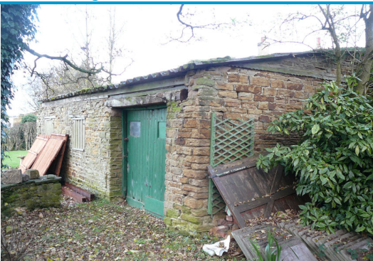
The former smithy, Craig House – stone and originally pantiled roof, although now has a replacement corrugated sheet roof
