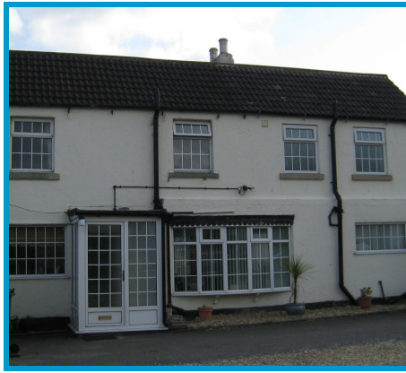
Inappropriate rendering of stonework at Stud Farm
