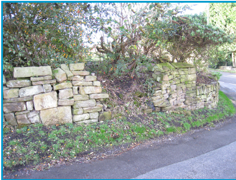
Boundary wall in poor condition at The Green
