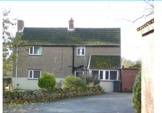
The Cottage, Pipes Farm – rendered façades with concrete tile roof and modern windows
