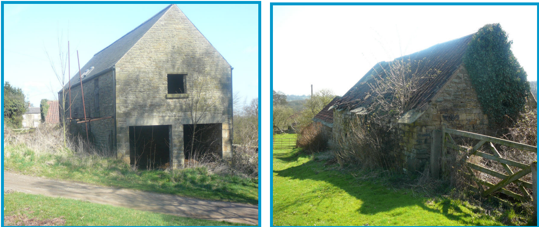
Buildings at risk in Astwith
