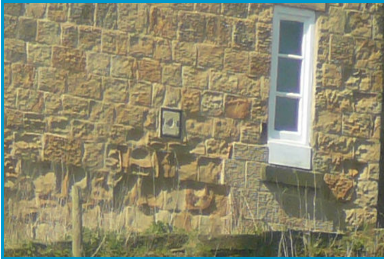
Example of eroded coal measures sandstone and repair work
