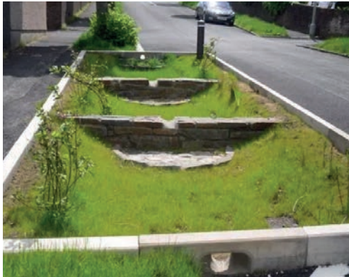
Linear street SuDs Swales.
